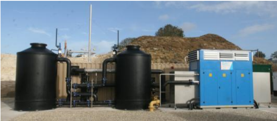
Figure 9: Carborex ® MS system for 650Nm 3 /h at Poundbury (UK)
